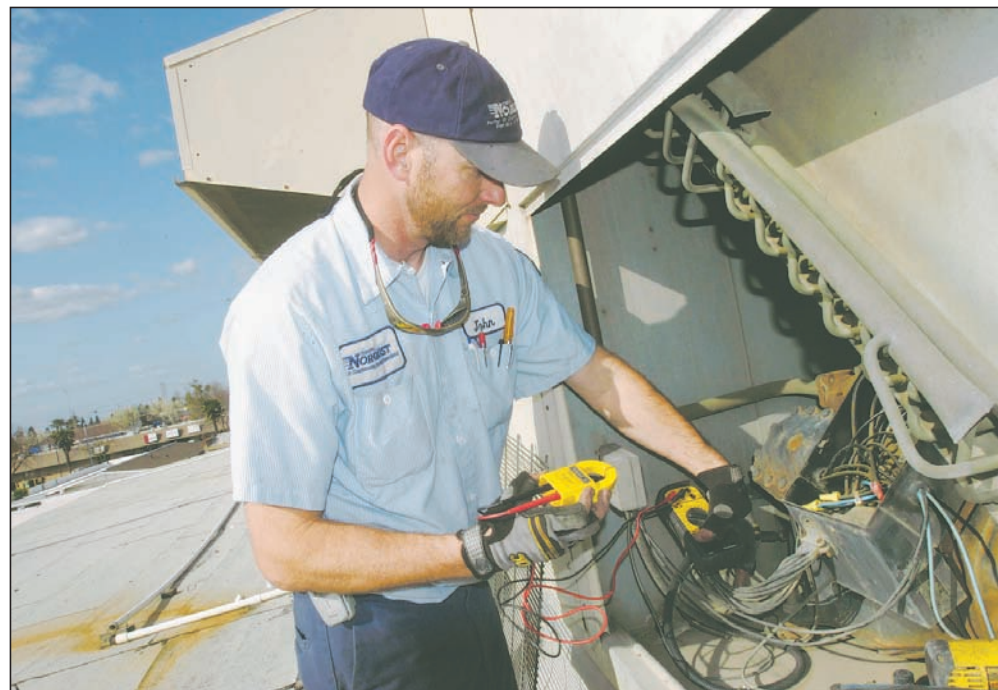
John Schulz, a certified HVAC technician with Tenney A. Norquist Inc. in Modesto, performs a preventative maintenance inspection on a commercial air conditioning unit. Schulz, who used the G.I. Bill to get his two-year certification and an associate degree from San Joaquin Delta College, has been repairing HVAC systems for seven years, since right out of school. An "endless amount" of available work offers job security, he says.
